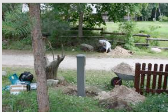
Fig. 34. Counters are installed at Mazirbe, 2010
